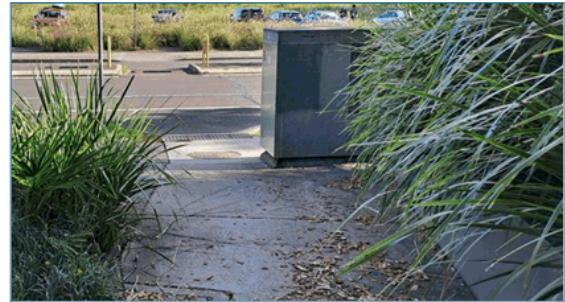
Looking back across Bennelong Parkway from western path, with NBN cabinet partially obscuring path and bark mulch on pathway.
