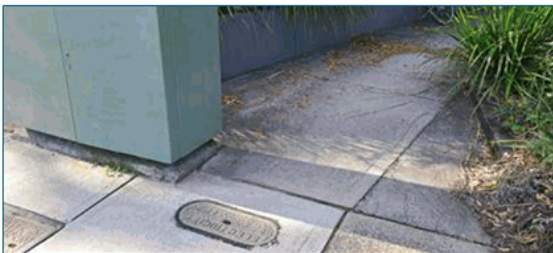
Extra concrete apron added to widen western path around the NBN cabinet.
