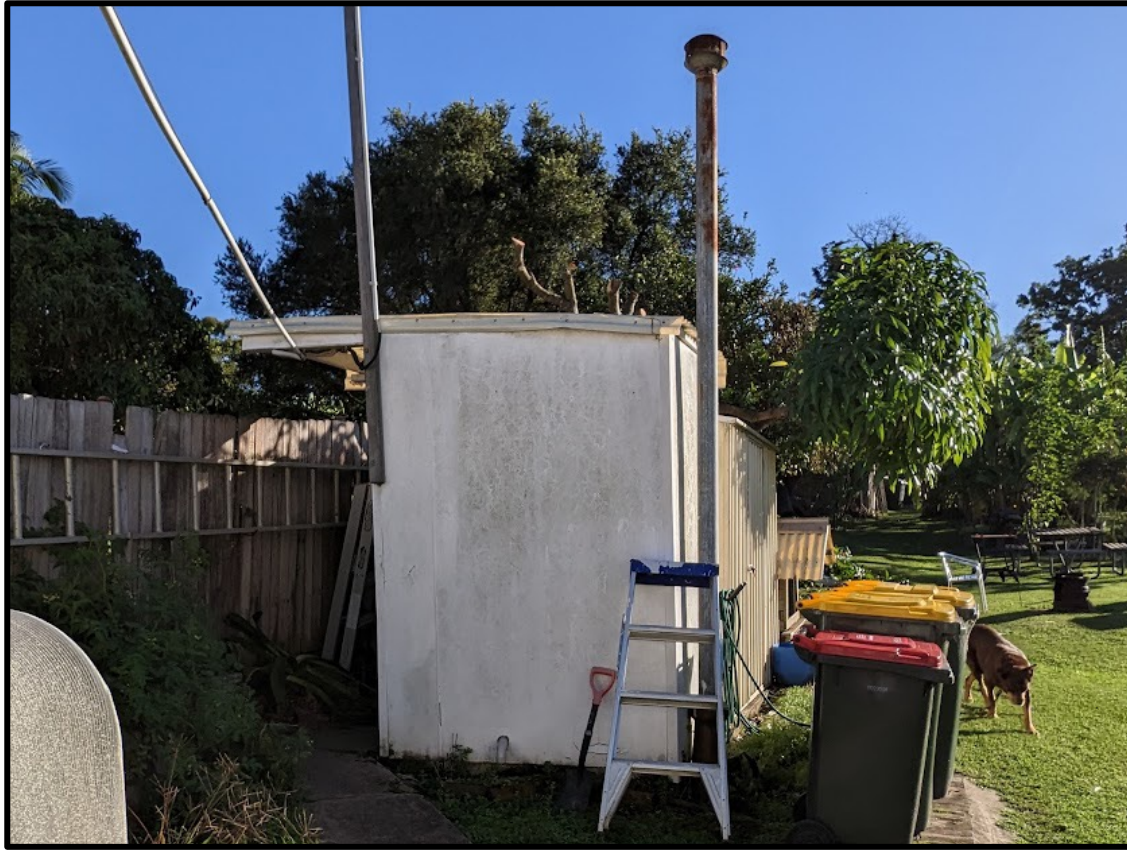
Figure 11. Fibrocement shed and swear plumbing air vent within the western portion of the site.
